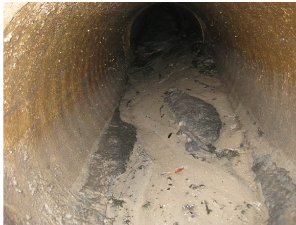
c. Accumulated Solids in Outfall Pipe
