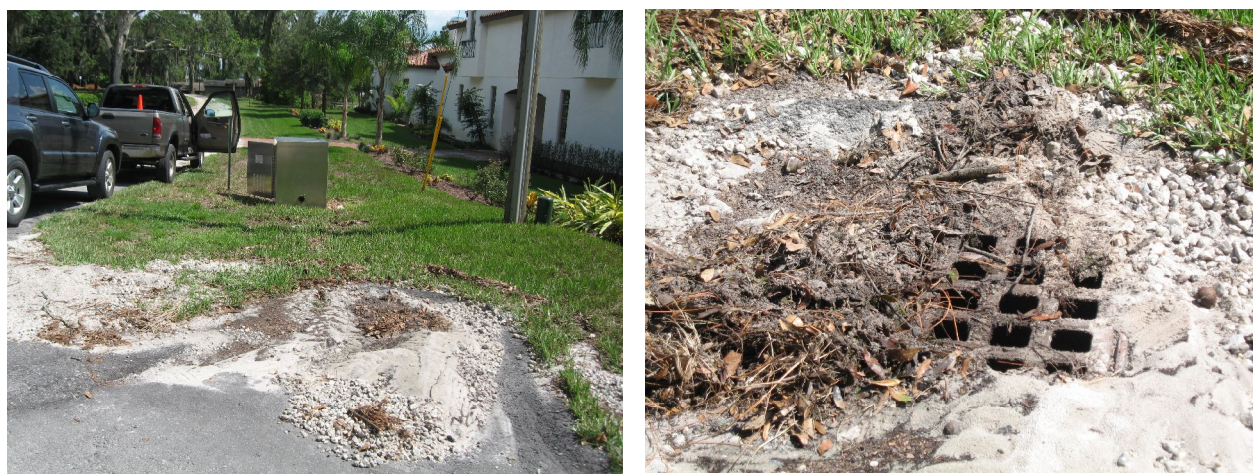
Figure 3-15. Accumulated Solids and Debris Around the Pine Street Stormceptor Grate Inlet.
