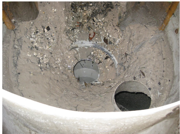
b. Accumulated Solids on Top of Stormceptor Unit
