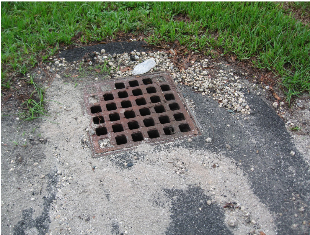
Figure 1-11. Photograph of the Inlet Grate Cover for the Pine Street Stormceptor Unit.
