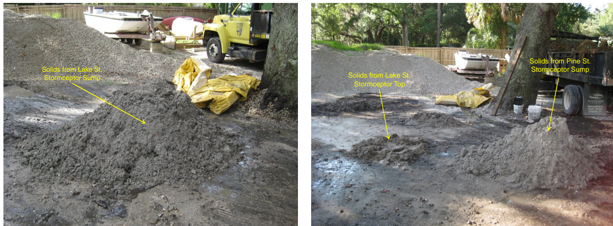
Figure 3-10. Accumulated Solids Removed from the Stormceptor Units.
