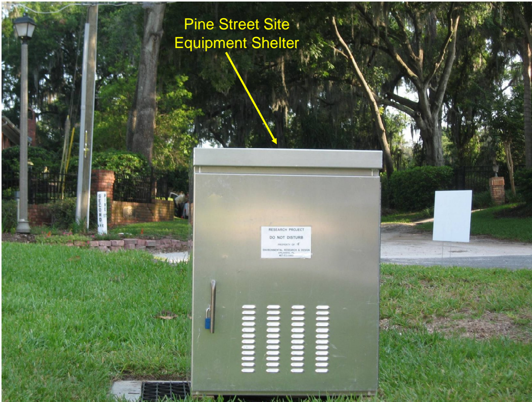
a. Equipment Shelter
