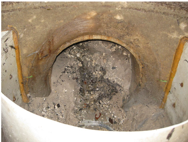
a. Inflow Pipe to Stormceptor Unit
