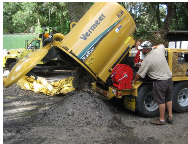
c. Solids Deposited at Town Storage Yard
